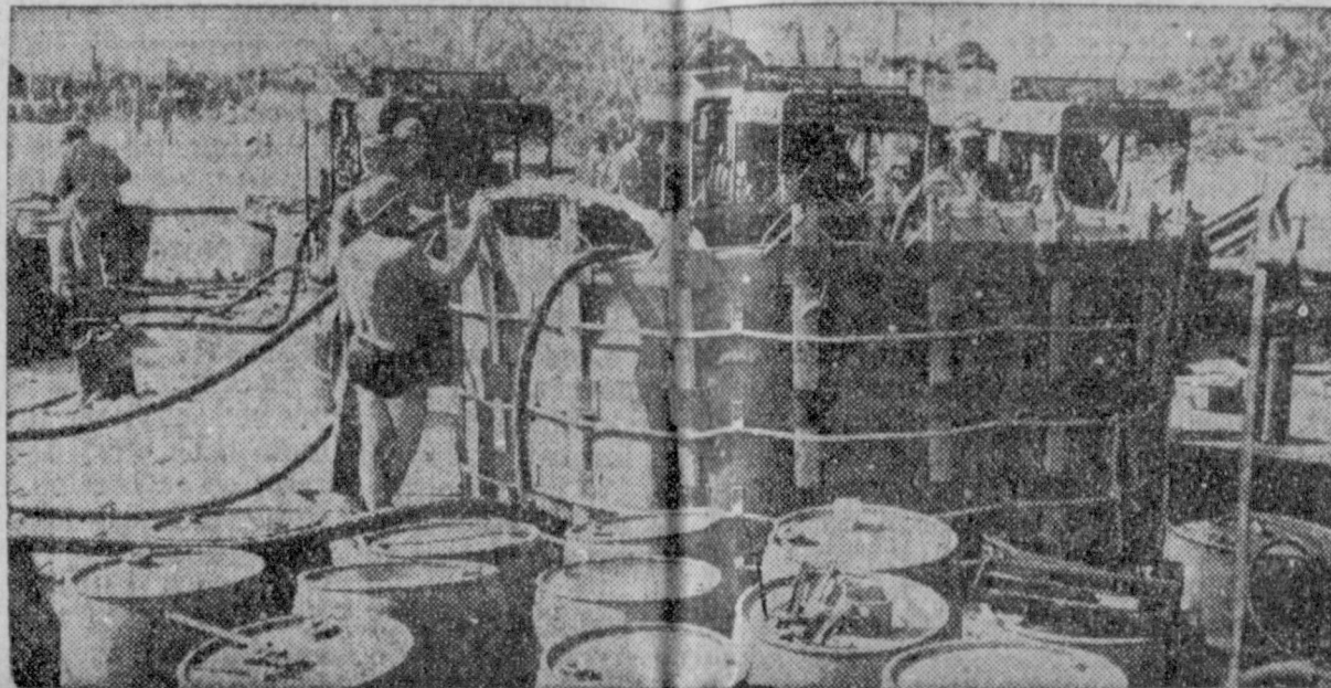
WATER'S PURE —Yanks fighting in the Marshalls don't have to worry about water. It's pure and plentiful, thanks to system installed on Kwajalein. Photo shows salt sea water being pumped into huge distillation storage tank where it is processed into fresh water.
