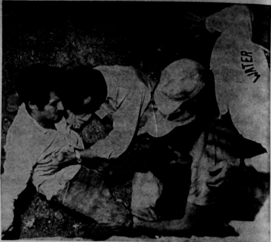
BRUSH WITH DEATH —Joe Vasquez is shown as rescue workers succeed in digging him from beneath several feet of dirt, under which he was buried Wednesday, May 15. Vasquez was working in a sewer ditch near the intersection of 1st and Geneva streets, when the cave-in occurred. Workers had uncovered his head when the walls of the ditch gave way, burying him for a second time. Members of the Slaton Volunteer Fire Department were summoned and finally were able to remove the man from the dirt. He was apparently uninjured.
