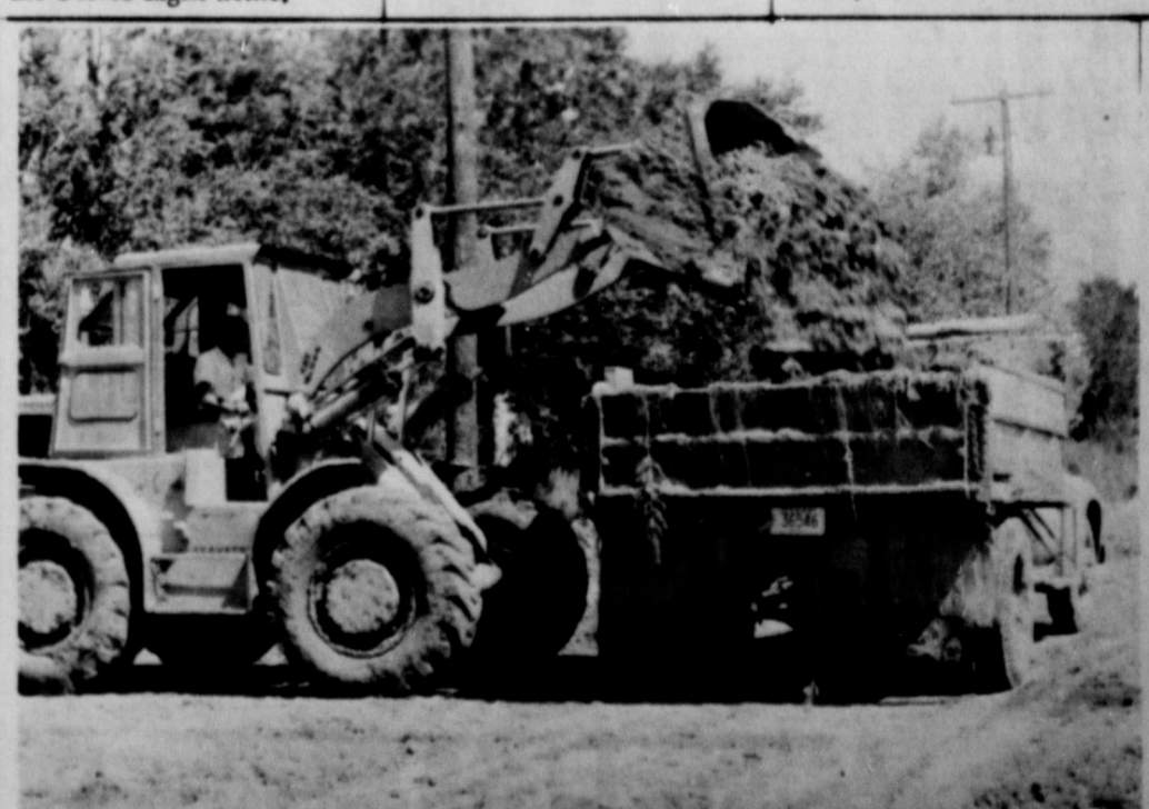
COUNTY CREW CLEANS UP... after the heavy rain Saturday night washed mud onto dirt roads over the area, causing the roads to be closed for a time. This picture was made three miles west and two miles north of Earth.
