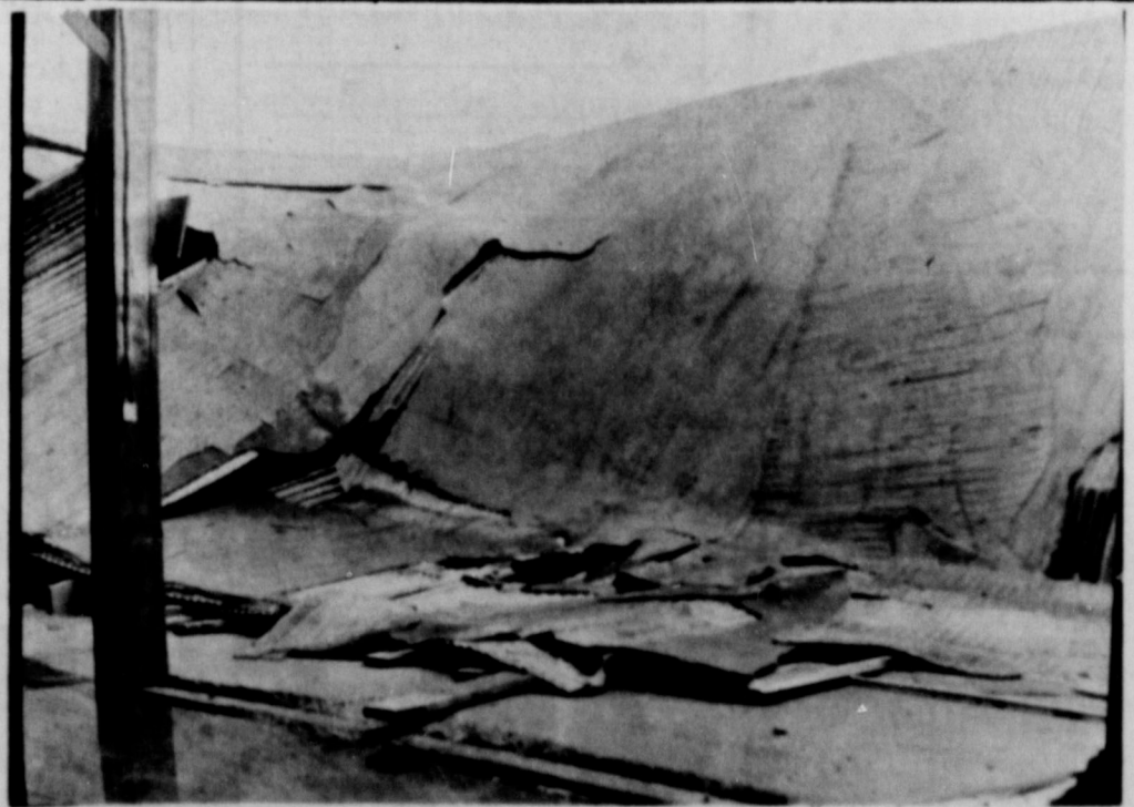
THE BUILDING FORMERLY OCCUPIED BY BROWN-WHITE EQUIPMENT was extensively damaged by high winds during the thunderstorm Saturday night, around 3 a.m. when the roof was blown off, and one side of the building caved in. The building was used as storage by the company, and several tractors were housed in it at the time, but were not damaged.
