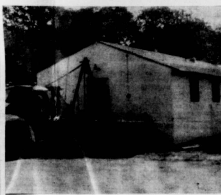
OUT WITH THE OLD - To make room for the new City Hall and community room, the old Lions Club building is being moved out by section this week.
