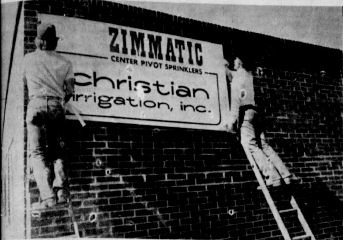
FINISHING TOUCH, Doug Campbell and Bailey hang the sign that signals the completion of the new facilities of Christian Irrigation. Doug Campbell is the manager for the office in Earth and Charlie is the service manager. The new facility offers complete sales of Zimmatic Irrigation systems and service and parts for all makes.
