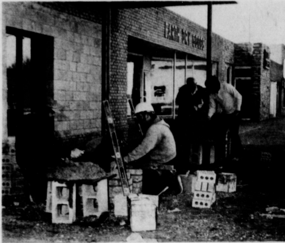
LOOKING BETTER EVERY DAY... Bricklayers were busy getting things ready to start pouring the sidewalk on the new bank expansion program.
