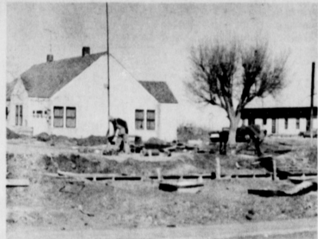
SITE OF NEW SPRINGLAKE SCHOOL CAFETERIA--Workers are busily preparing foundation forms as construction on the cafeteria moves along at a steady pace. It is hoped to have the structure ready for the fall term.
